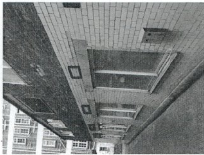
4 View of External Elevation Fitness Suite Intake and Discharge Louvers
